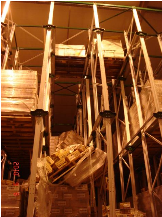
No.9 Deflected columns to drive-in racking.
