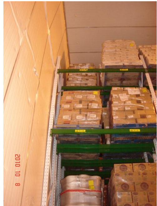
No.12 Wall pounding of double deep selective racking.
