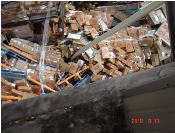
No.17 Collapsed double deep racking.
