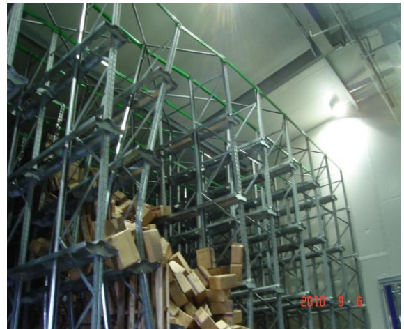
No.16 Deflected columns to drive-in racking.
