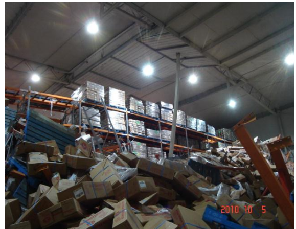
No.17 Roof prop impact from collapsed racking.
