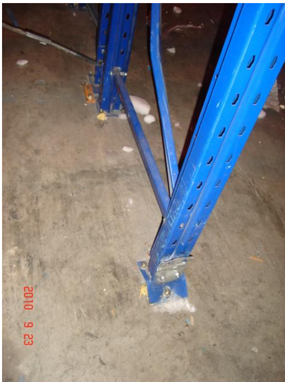
No.8 Baseplate & brace yielding to columns.
