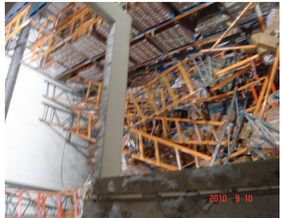
No.17 Collapsed drive-in racking.
