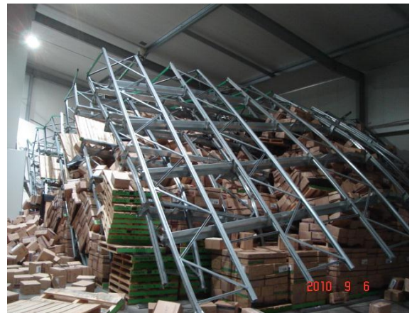
No.16 Collapsed drive-in racking.
